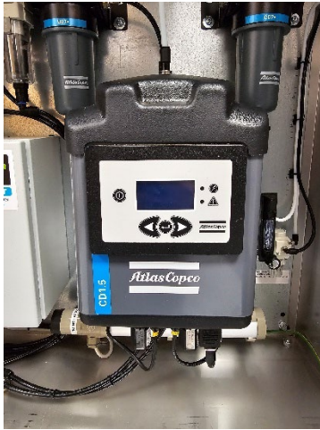
Figure 37: CD1.5 desiccant dryer
