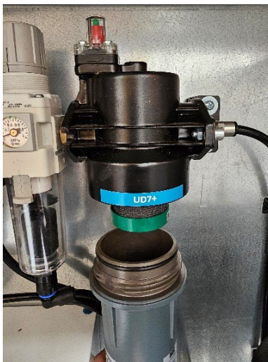
Figure 21: Filter bowl removed showing old UD7+ filter
