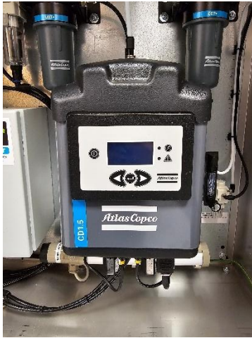
Figure 37: CD1.5 desiccant dryer
