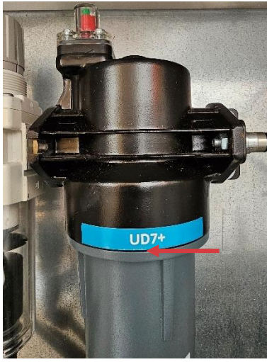
Figure 26: Filter bowl fastened with no gap at seam
