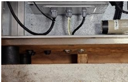
Figure 33: Exhaust silencers location
