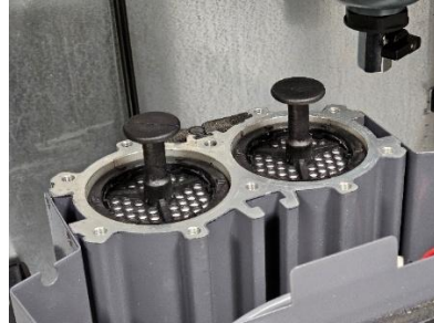
Figure 42: Removed cap reveals desiccant cartridges
