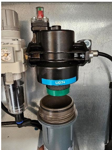
Figure 21: Filter bowl removed showing old UD7+ filter
